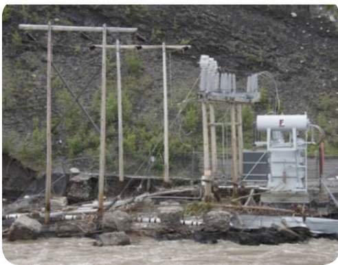
Figure CS1.1 The flood-damaged Barrier 32S substation, June 2013 5
